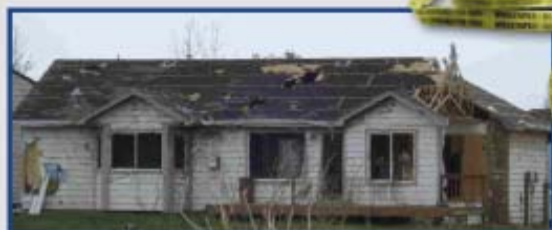
* Photo of Windsor, CO home with shingles blown off and tarpaper, installed with Windstrips and staples, remaining after F3 tornado.
