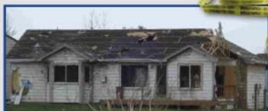
* Photo of Windsor, CO home with shingles blown off and tarpaper, installed with Windstrips and staples, remaining after F3 tornado.
